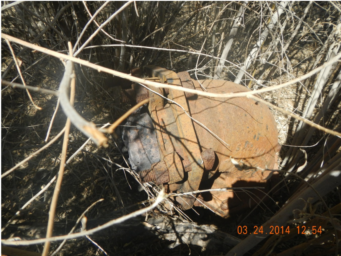
Figure 1: Iron pipe elbow rising from the ground surface in the Topock 1 area in Arizona.
